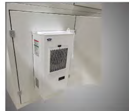
Electrical cabinet air conditioner
